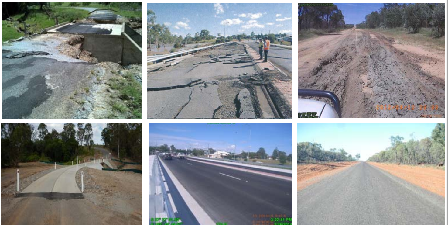
Projects undertaken with Betterment funding — event damage (top) and post completion of works (bottom) - (left to right): Cherry Tree Road (Fraser Coast Regional Council), One Mile Bridge (Ipswich City Council), Richmond Road (Croydon Shire Council)
